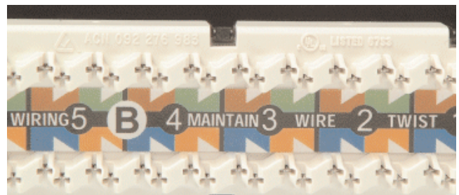
Close up of the rear of a 6-port module showing the label and wiring configuration
